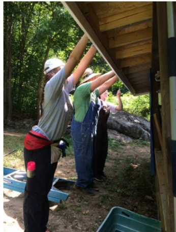
Above: Youths Gabi Huston and Zayne Ireland hold up part of the roof so Annie Sherrick can drill it into place.
